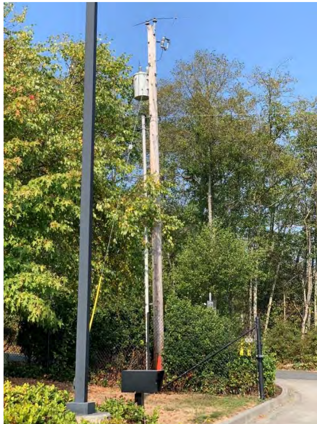
Figure 7 Service Transformer at the Camano Island Storage Facility
