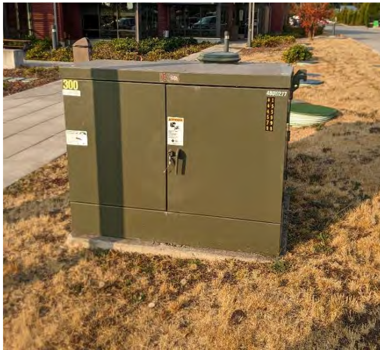
Figure 6 Whidbey Island Coupeville Facility Distribution Transformer
